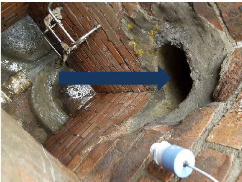
Figure 2-2 : COP showing high level overflow to stormwater (arrow), and water level monitor.
