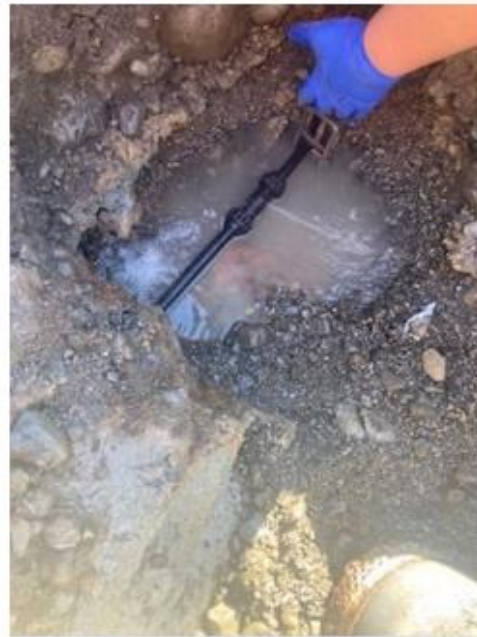
Photo of service leak taken by repair team on 15/9/2022
